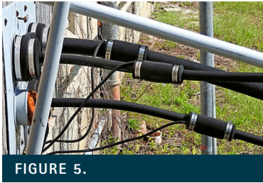
The shield of the coax going to the tower is bonded to the external grounding bar by means of Andrew's Cuffs. The majority of lightning energy on the shield is thus diverted to the extensive external grounding system, rather than the internal equipment where it can do damage.
