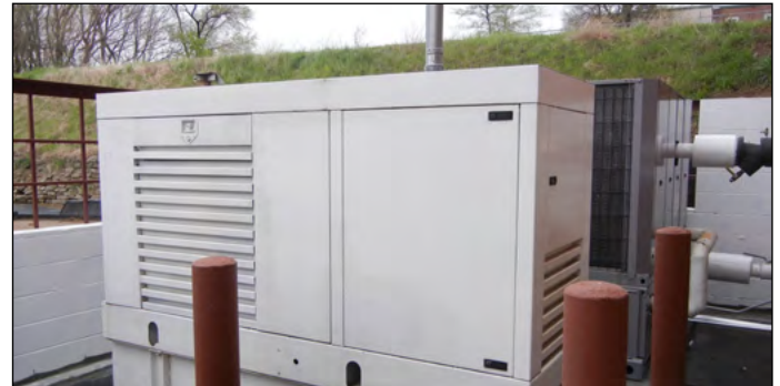
Figure 1. The LoCoCoLo data center has one 80-kVA generator and an associated UPS, but the facility is located nearby a utility grid cross-breaker. A grid outage on one side of the breaker can be re-routed to the center within an hour, and the generator shown above has a four-day fuel capacity.
