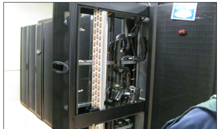
Figure 2. An in-row cooler shown ready for installation between two server stacks. Placed near the heat source, the rapid response, copper-coil coolers operate with 30% greater efficiency than conventional peripheral cooling system, a major energy and cost savings.
