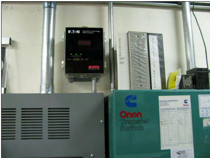
Figure 3. The black-colored surge protection device (SPD) mounted atop the LoCoCoLo service entrance cabinet protects the center from surges as high as 300 kA. It is very important that SPDs are securely bonded to a robust, low-resistance, single-point grounding system. Without proper grounding, SPDs cannot function properly and will not protect the electrical system on which they are installed.
