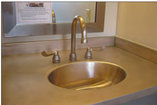
Figure I-3. Antimicrobial Copper sink and faucet installed at the Ronald McDonald House of Charleston, South Carolina. Healthcare facilities around the world are recognizing products made from EPA-registered Antimicrobial Copper alloys continuously kill bacteria that cause infections. The sink is made by Elkay Commercial Products and the faucet by Rocky Mountain Hardware.
