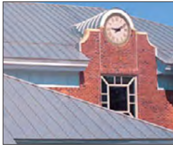
Figure II-3. The pleasing, naturally weathered, soft gray color on this roof and dormer is provided by lead-free, tin-zinc coated copper from Revere Copper Products.
