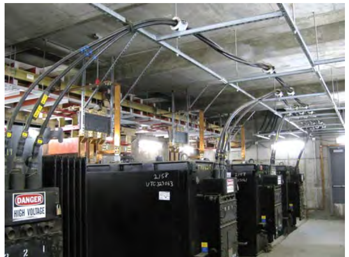
Figure 3. Four of eight 13.8 kV-480 V utility transformers located in a vault at One Summer Street. A similar set of transformers in a separate vault form the other half of the double-ended utility feed. Copper buswork seen at the upper left feeds distribution switchgear located in the basement. Utility ground straps are visible on the floor and rear wall.
