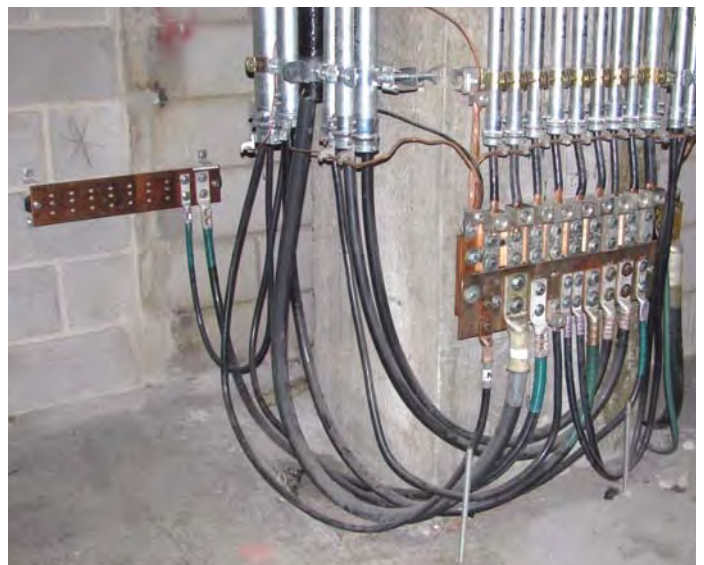
Figure 7. The main grounding bar at One Summer Street is a three-foot by one-foot copper plate (right) located in the subbasement. All grounding conductors in the building's two grounding system branches terminate here. The smaller bar at left rear is an extension of the larger bar.
