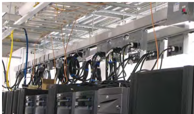
Figure 6. Power is fed to equipment cabinets via power distribution units (PDUs), seen here. Each PDU/cabinet is served by a minimum of two branch circuits providing 2N redundancy. Copper grounding conductors are run in ladder racks, above.
