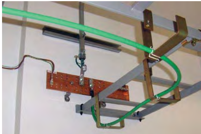
Figure 10. Multiple grounding collector bars are mounted on walls in server rooms. The AWG 2/0 conductor, top, leads to the riser bar, while #2 green cable, bottom, is a collector bus for a row of cabinets. Conductor sizes vary with clients' needs.
