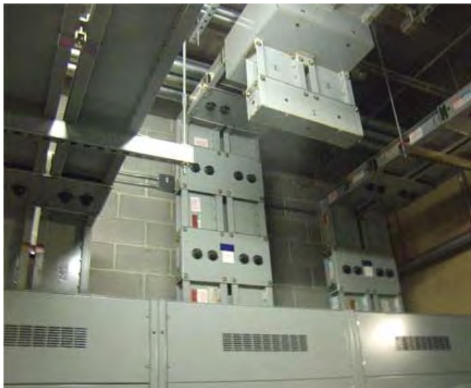
Figure 4. Switchgear (in cabinets, bottom) and three of the ten 480-V, 4,000-A copper bus risers that feed power to upper floors (top of photo). Four 5,000-A bypasses enable switching among primary feeds.
