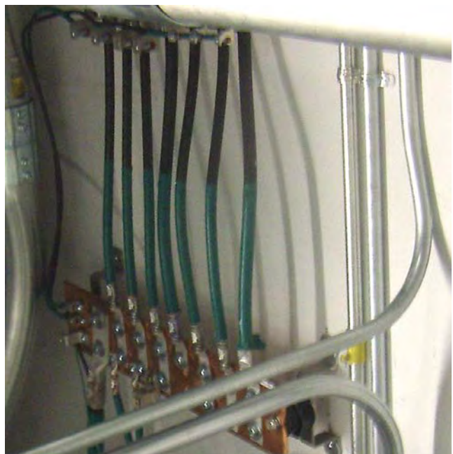
Figure 9. A 1,000 kcmil grounding conductor (lower left) from the main grounding bar terminates at a ground bar serving one floor from one of the building’s two ground risers. Smaller conductors bonded to the main floor bar (upper cables) lead to collector bars on the floor.
