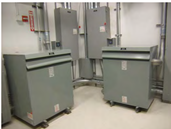
Figure 5. Two (of more than 100) redundant 480 V-208/120 V distribution transformers feed customers’ servers and convenience outlets. All sub-distribution transformers are copper-wound, dry-type, K-rated, and meet NEMA TP-1 efficiency standards.
