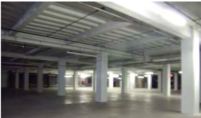
Figure 1. Fifteen-foot ceilings at One Summer Street enable installation of 24" to 36" raised floors while maintaining ample overhead space for cable trays and racks.
