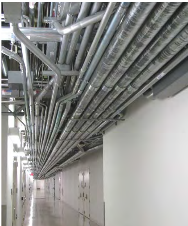
Figure 8. Typical conduit runs at One Summer Street illustrate why the center relies on separate internal green wires rather than conduit itself as the grounding path. Copper is a better conductor than conduit steel. And, if conduits were used for grounding, thousands of connections and fittings would have to be inspected, torqued and tightened periodically, a hopeless task.
