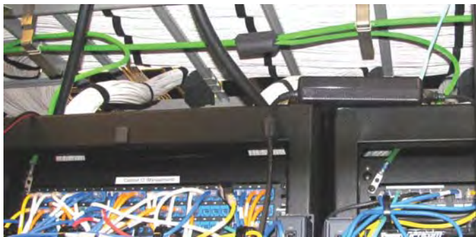
Figure 11. Green grounding conductors bond individual cabinets to an overhead collector bus. In this example, cabinet grounds are AWG #6 and the collector bus is #2, but larger sizes may be used.
